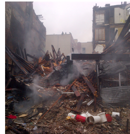
GAS EXPLOSION IN EAST HARLEM 2014
